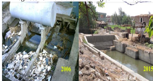
Fig. (10): The situation of the automatic gates in Dakalt canal during 2006 & 2015
